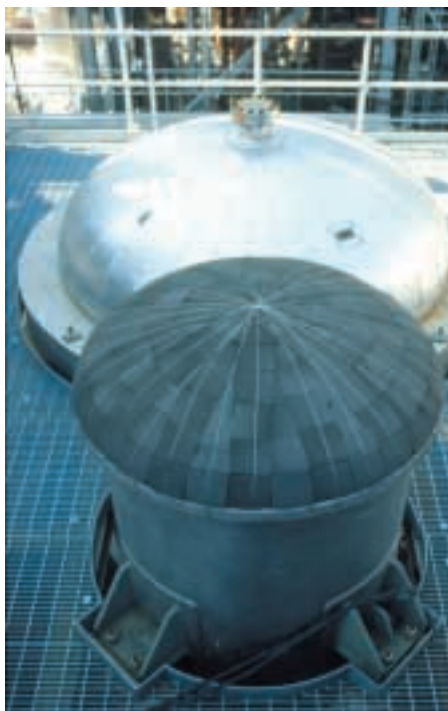
FOAMGLAS® Super K™ insulation was field fabricated for odd shapes such as vessel heads (as shown). For easier access, flanges, pumps, controls and other odd shapes were covered with hard insulation boxes constructed of aluminum and FOAMGLAS® Super K™ insulation.
