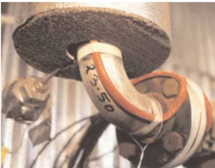
About 80 percent of the plant's piping system is equipped with either electric- or steam-heat tracers. Throughout the manufacturing process, system temperatures vary from -150° to 600°F.
