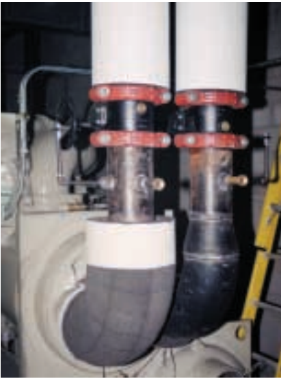
To protect thermal efficiency, chilled water supply and return lines are covered with 2½ inches of FOAMGLAS® insulation.
